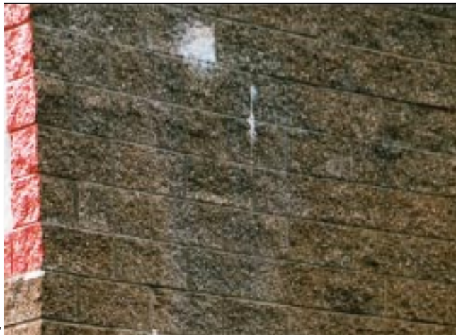
Days after a water-based water repellent made from concentrate was improperly applied to on a concrete masonry building in Clackamas, Ore., dark streaks appeared where one coat overlapped and reacted with an adjacent coat.
